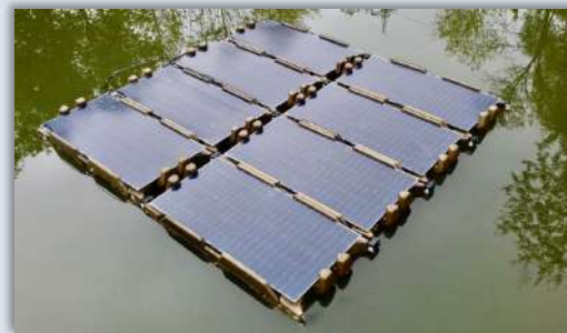
Floating solar panels SolOcean Vienna (Austria)
